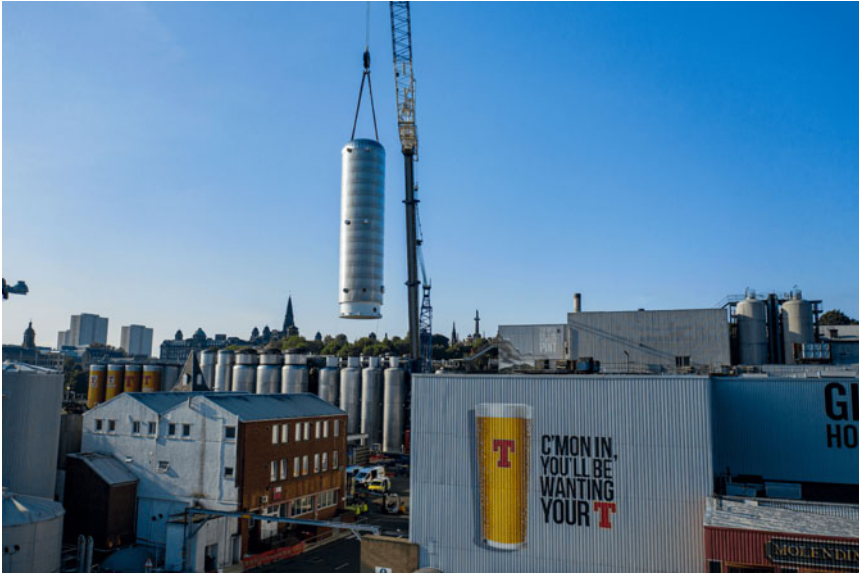
Figure 6: Part of the new CO 2 recovery plant being moved into place at Wellpark Brewery.
