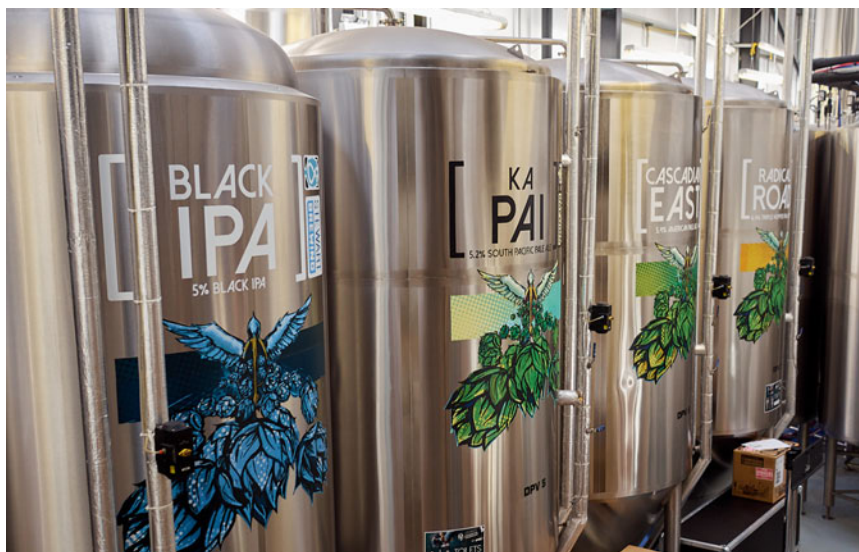
Figure 1: Tanks in situ at Stewart Brewing.
