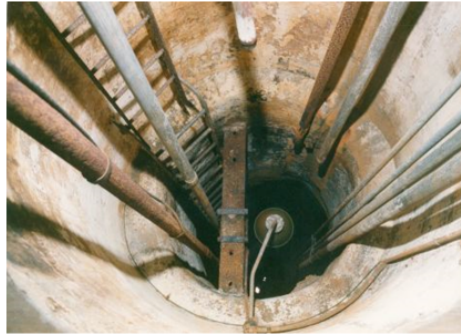
Figure 5: The interior of the brewery water storage well. This was not one of the two productive wells.
